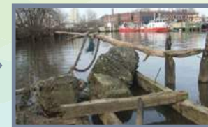
Infrastructure that ultimately fails and is not resilient to change
